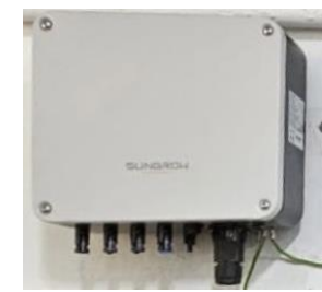
Battery Conjunction Box
