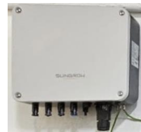
Battery Conjunction Box
