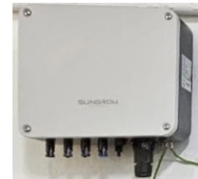
Battery Conjunction Box
